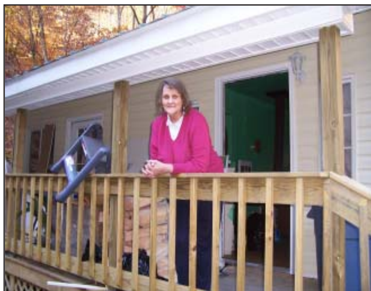
Lauda on her new porch with steps and a railing. Note the door and window frames, siding, and drain spouts.
